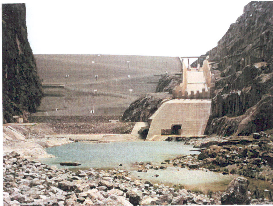
Fig. 2: Downstream view of the dam and the spillway chute with the dentated flip bucket and the tailrace plunge pool.
