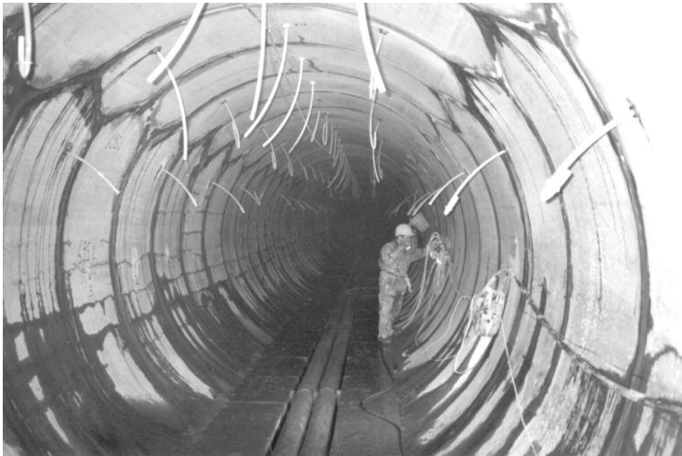
Figure 6: Progress of the grouting works without any mixing plant in the tunnel.
